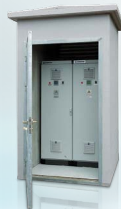
Two converters KONTRAC PN30AC installed in Drivenik Railway Station, Croatia
